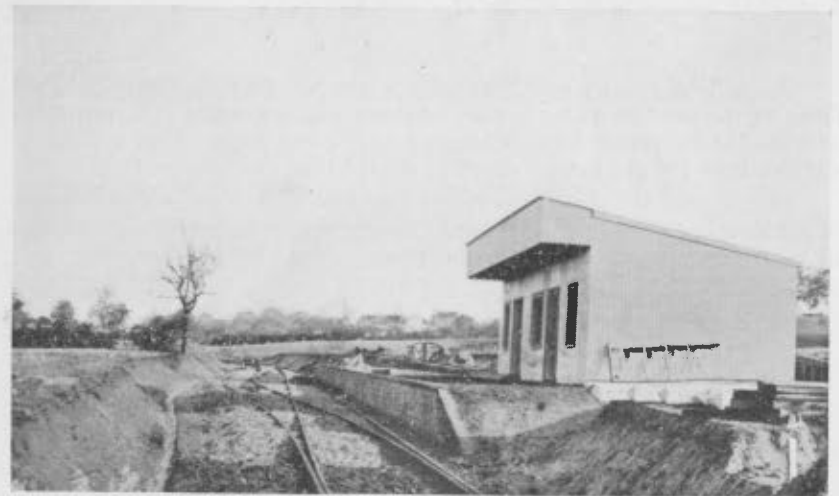
View taken when the line was under construction reputed to be Northiam Station. Resurrected from an old print in the possession of Mr. Dobell.
